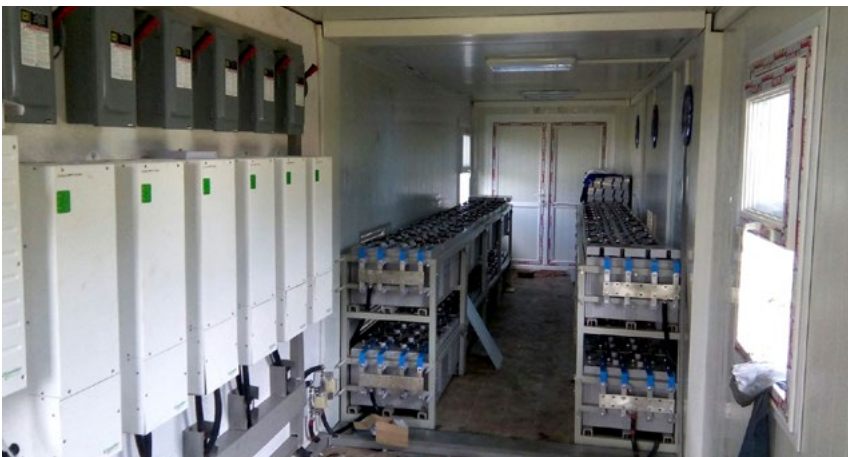
Interior view of solar powered container built with a modular system of battery-based inverters and charge controllers
