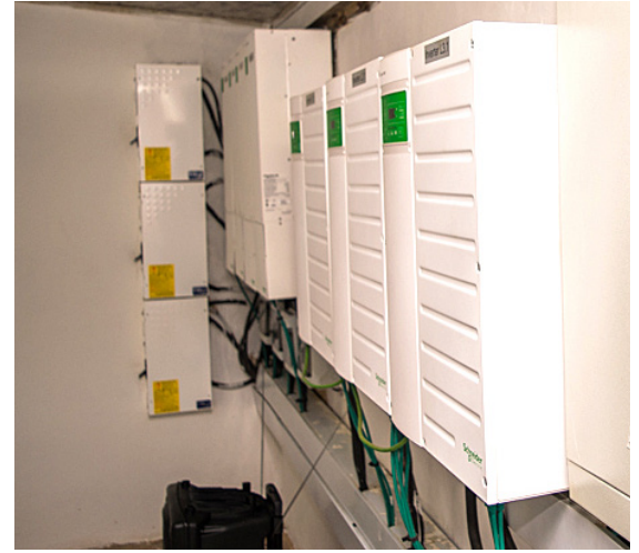
Kigbe Community, Abuja with 25kW Off-grid Solution.
